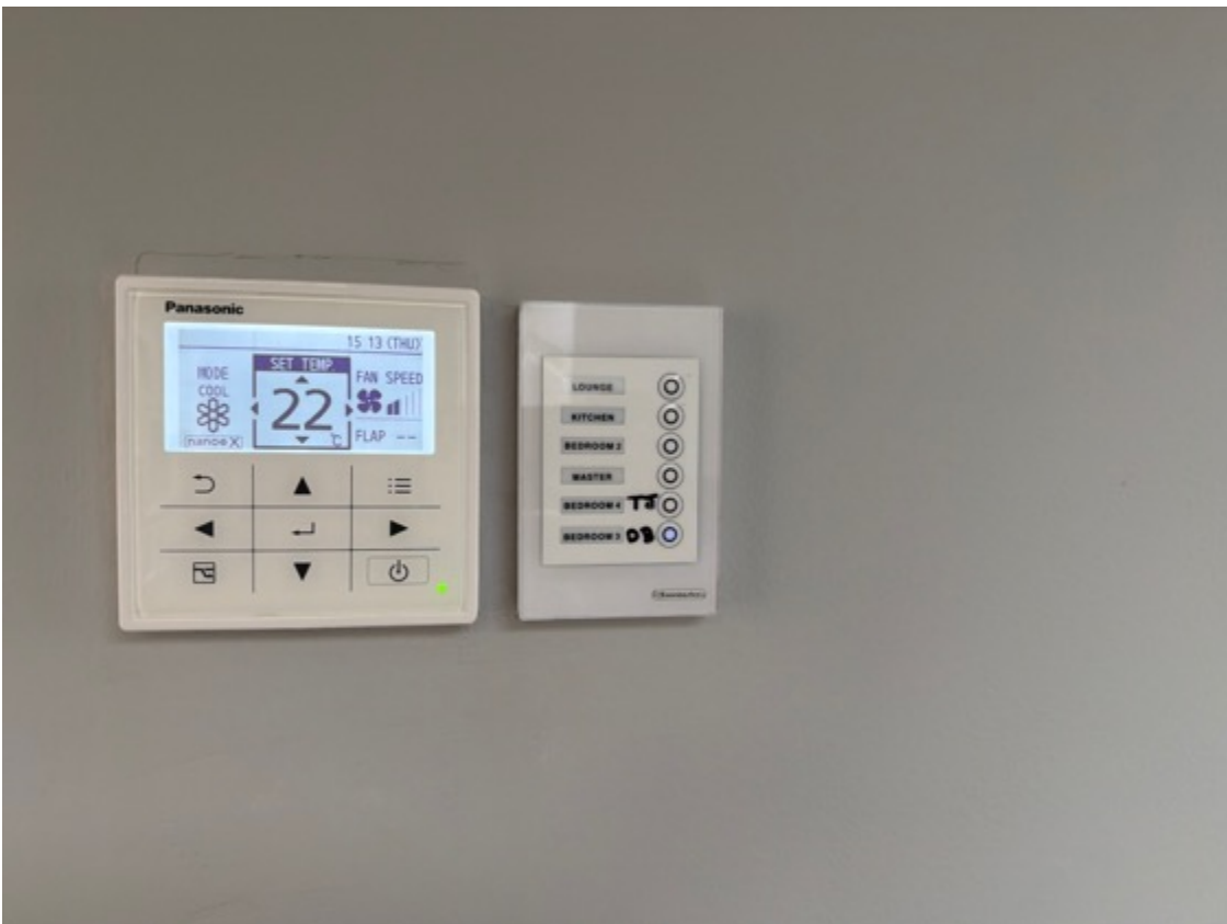
The AC tested, functioned at the time of inspection.
