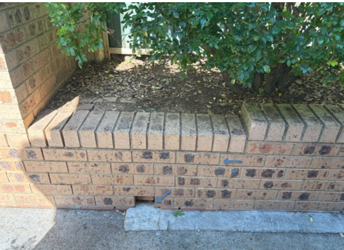
Isolated sections of external brickwork displays category one cracking, and one brick is missing here (front retaining wall example above.)
