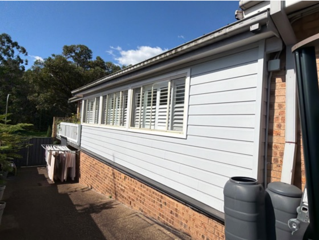
Exterior timber displays moderate level weathering and surfaces are paint blemished - consistent with age.
