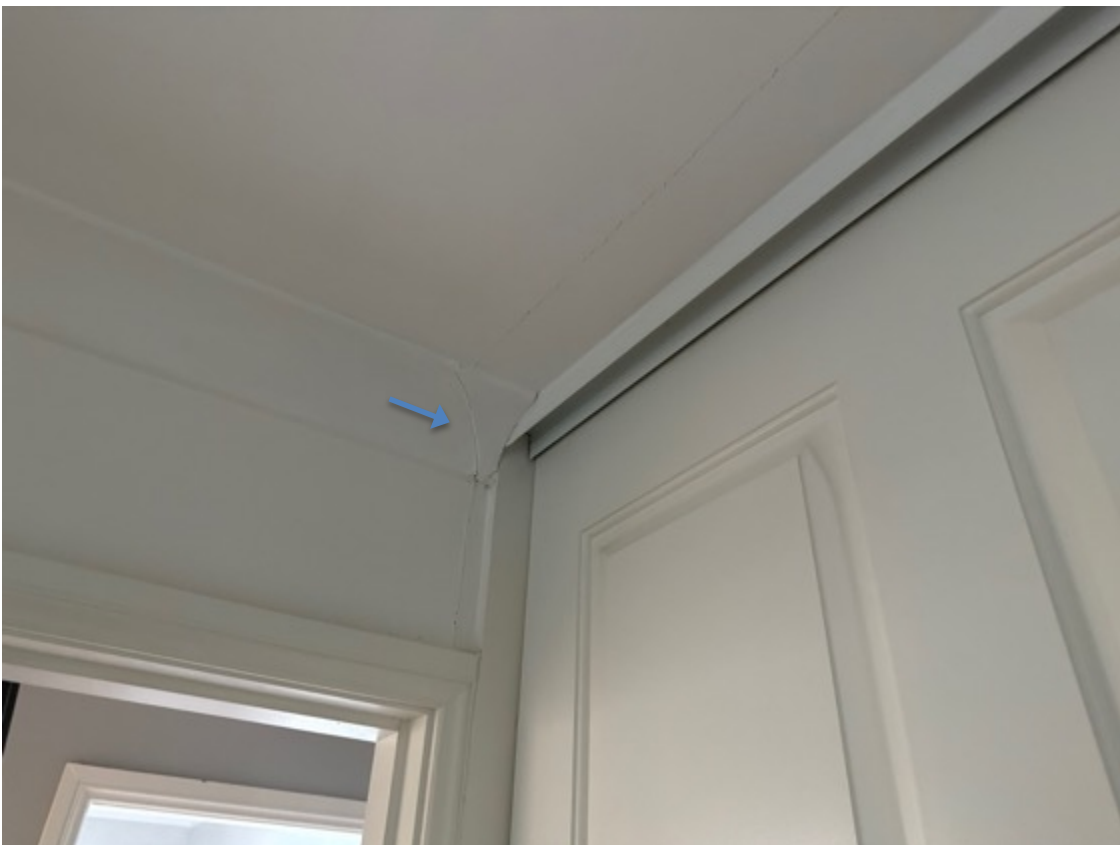
Isolated sections of plasterboard and cornices are cracking (mid left side bedroom area above.)
