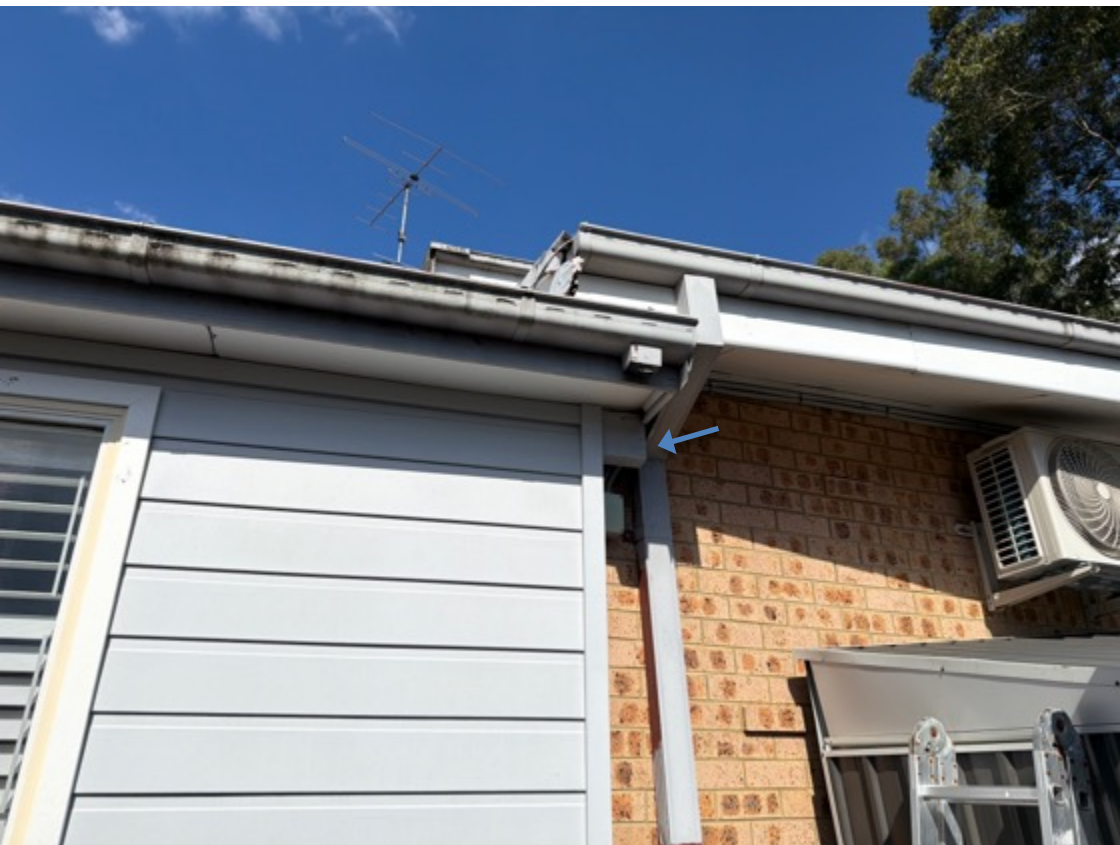
Example right side elevation rotten fascia board.
