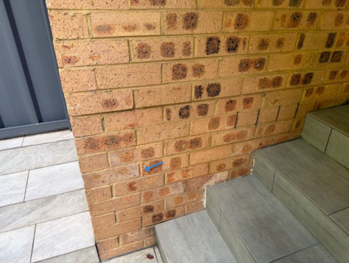
Front elevation example category one hairline cracks near the front entry door.
