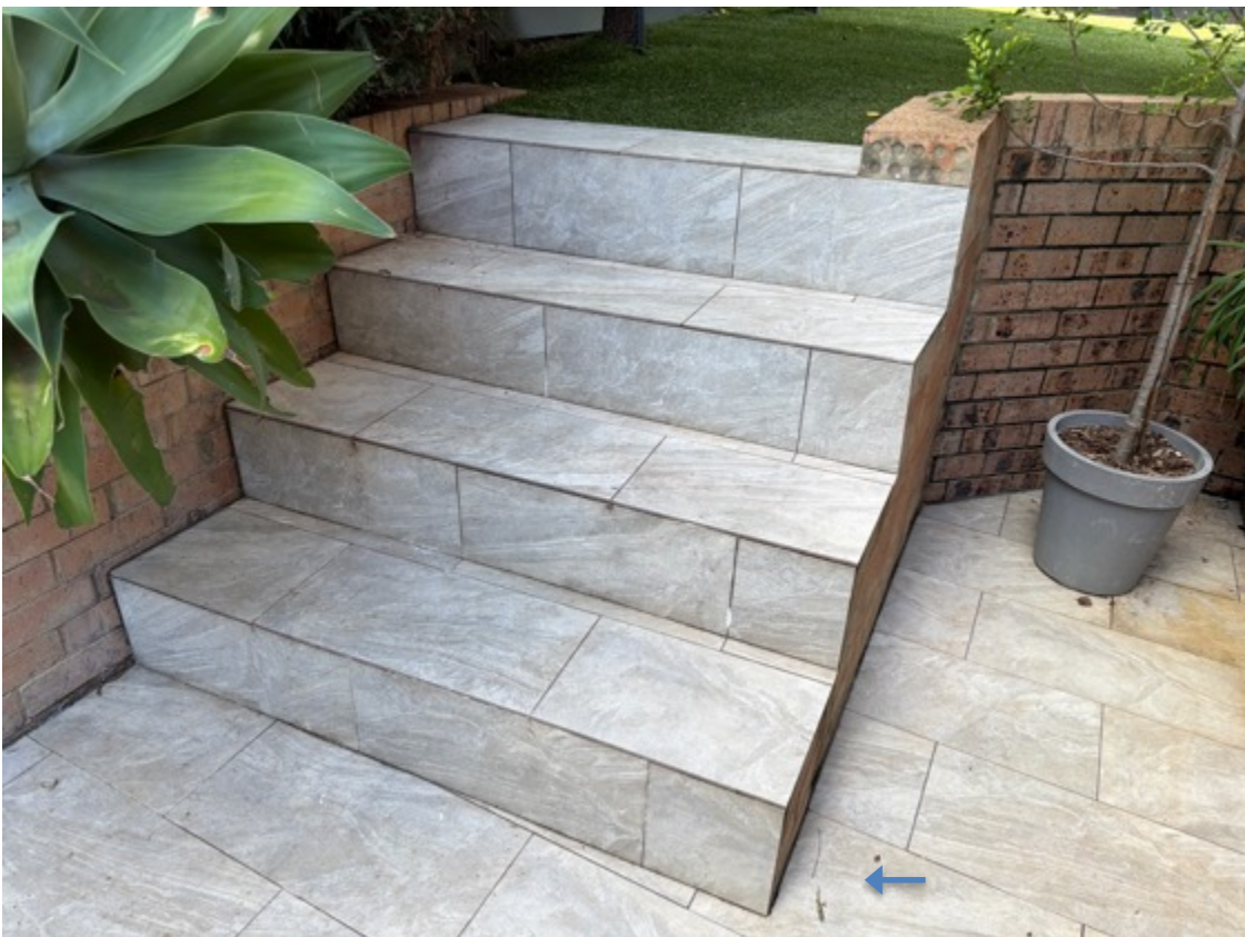
Isolated sections of external tiles are cracked and have minor efflorescence, consistent with age (front patio example above.)
