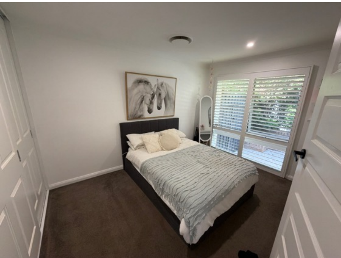
All interior lights tested, functioned as intended at the time of inspection.
