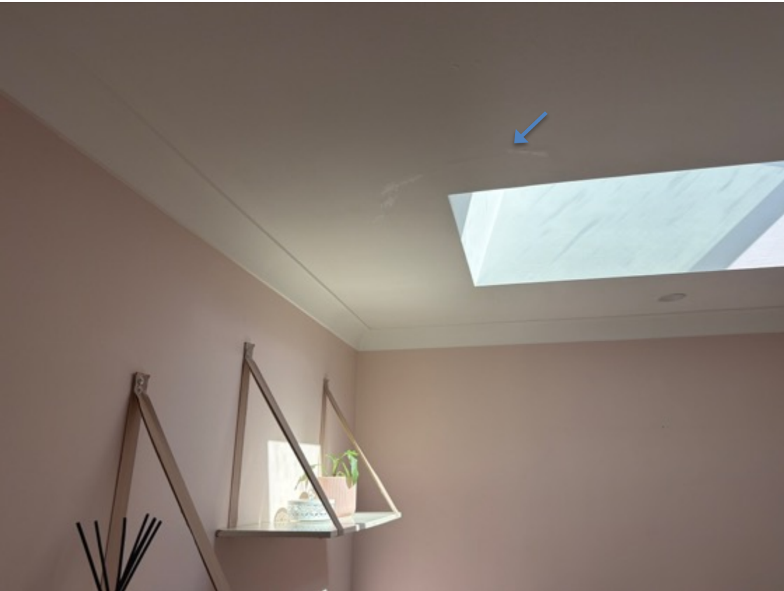
Plasterboard has minor water ingress visible here.
