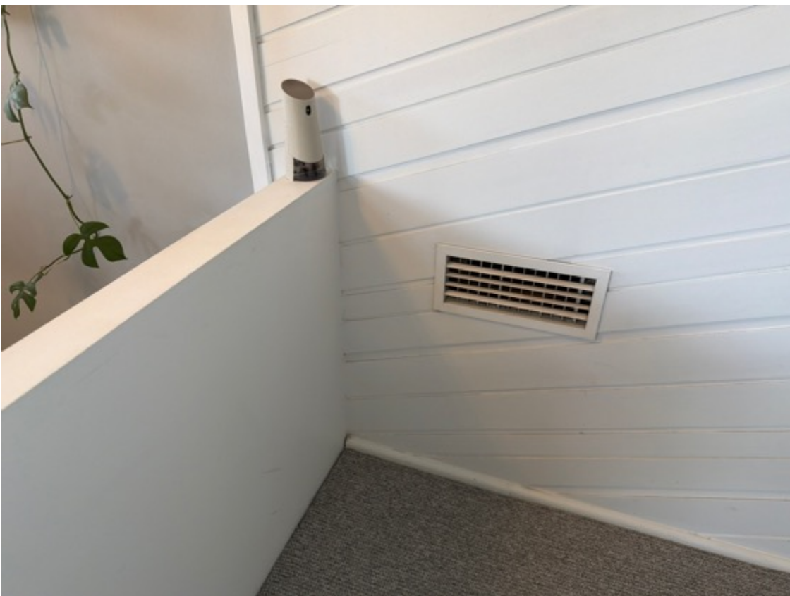
Surfaces display low level paint blemishes, consistent with age.
