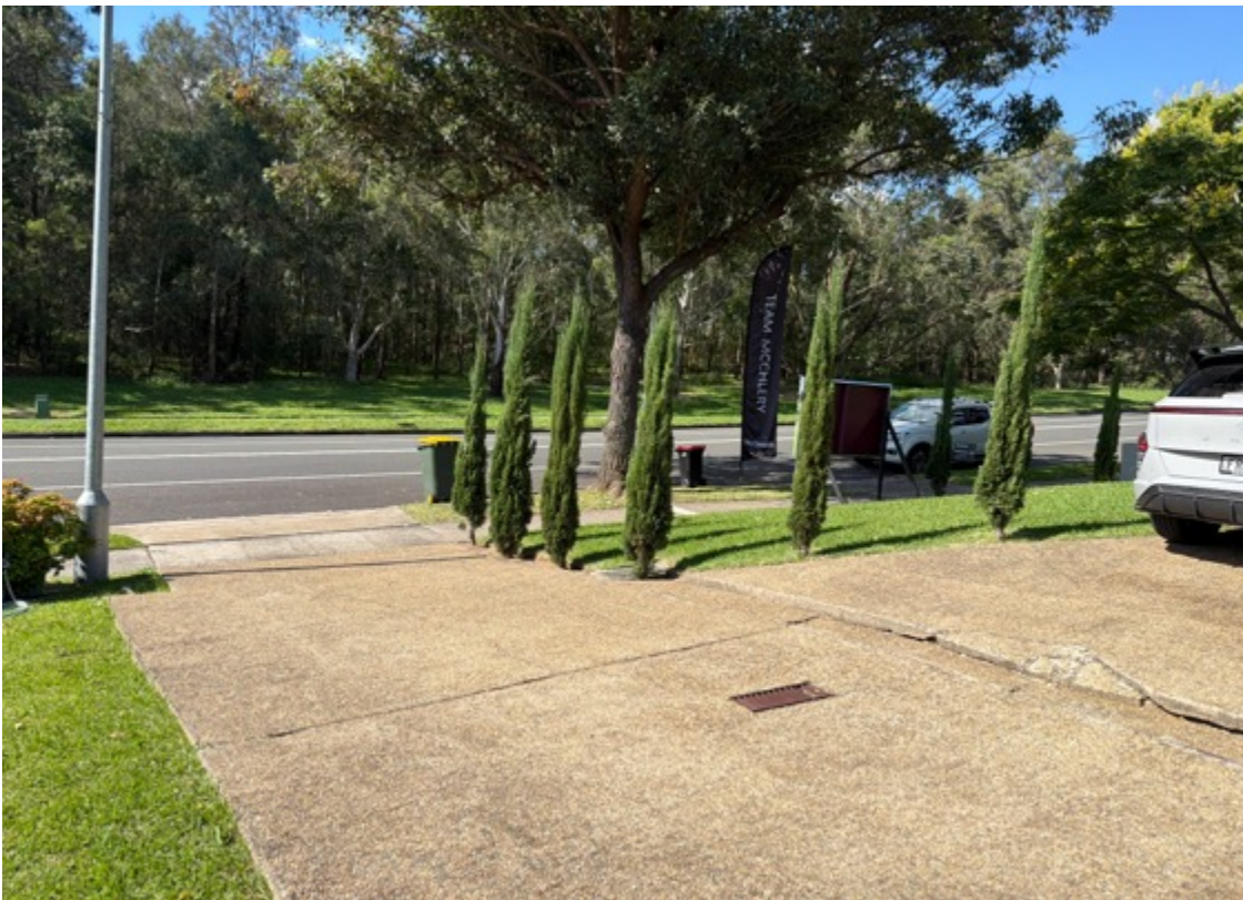
Exterior concrete presents in satisfactory condition for the age - isolated sections are cracked and undulating (consistent with age.)
