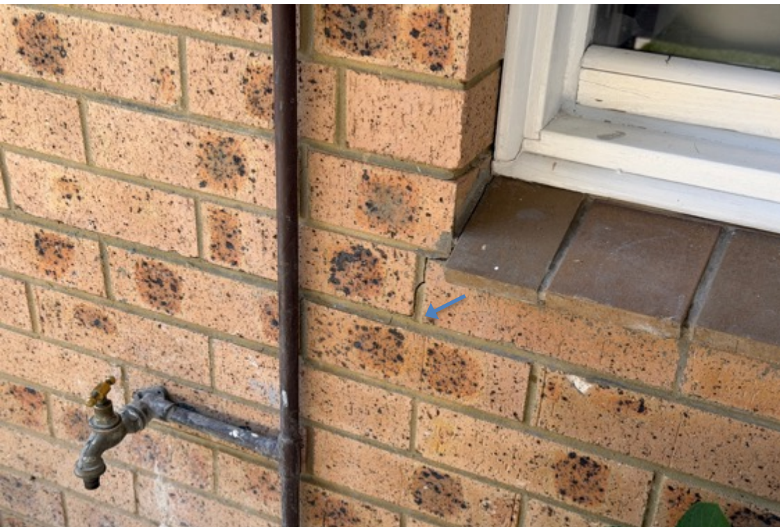
Example rear elevation cat one brickwork crack.
