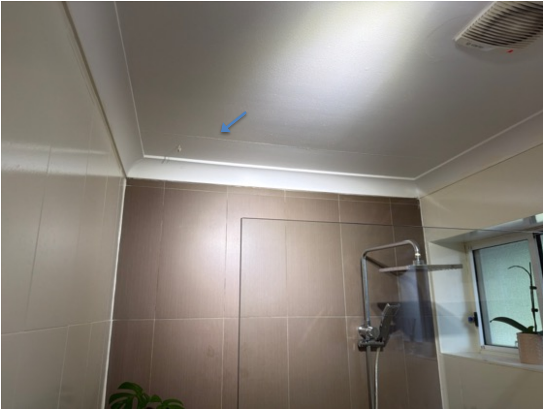
Plasterboard and cornices display imperfections - plasterboard has a crack above the shower here.
