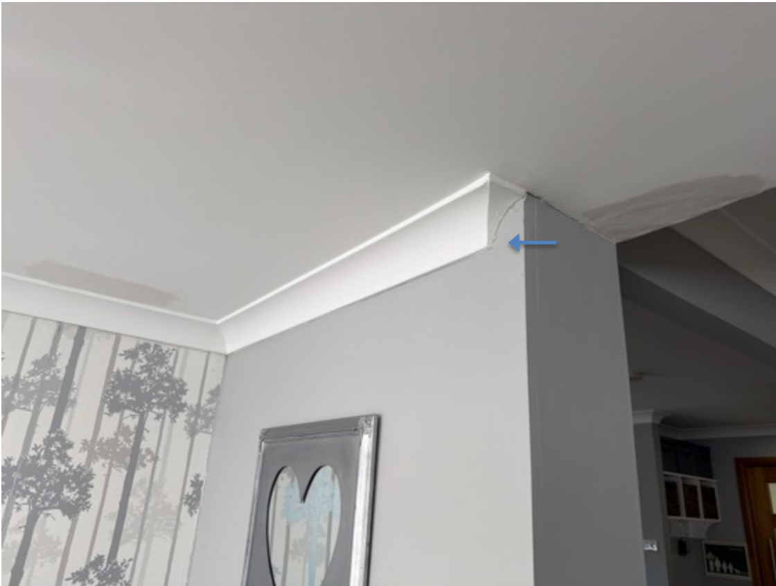
Sections of living area plasterboard has patches and cracks visible here.
