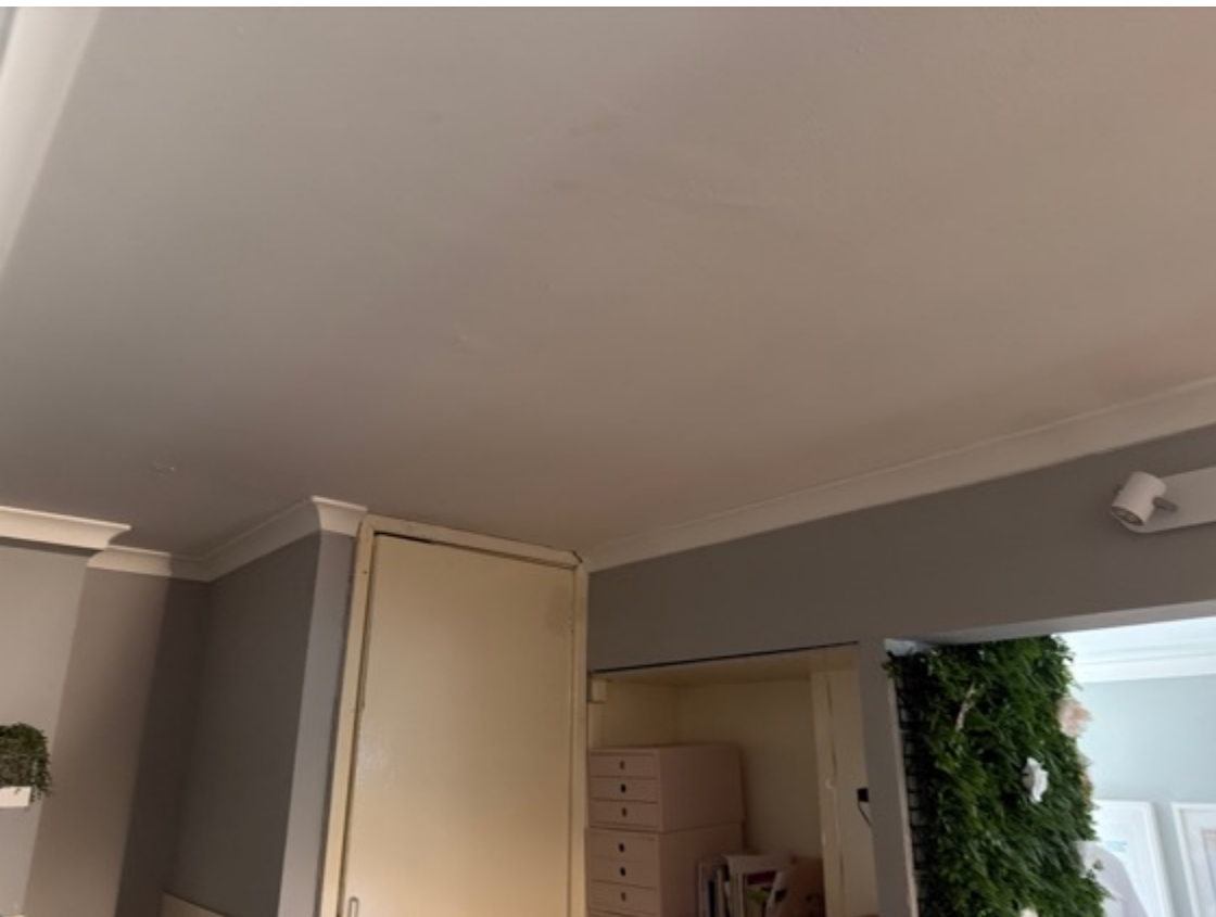
Plasterboard has minor patches and paint blemishes visible here.
